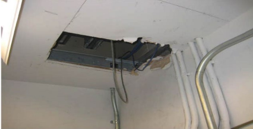
Whitman Center – breach in fire-rated ceiling assembly.
