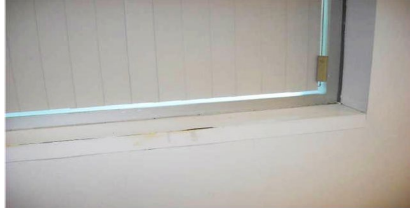
Whitman Center – water infiltration along exterior wall has caused deterioration of the plastic-laminated windowsills.
