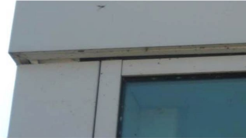
La-Z-Boy Center – It appears there is a void within the exterior aluminum, curtain wall assembly allowing the environment to enter the interior.
