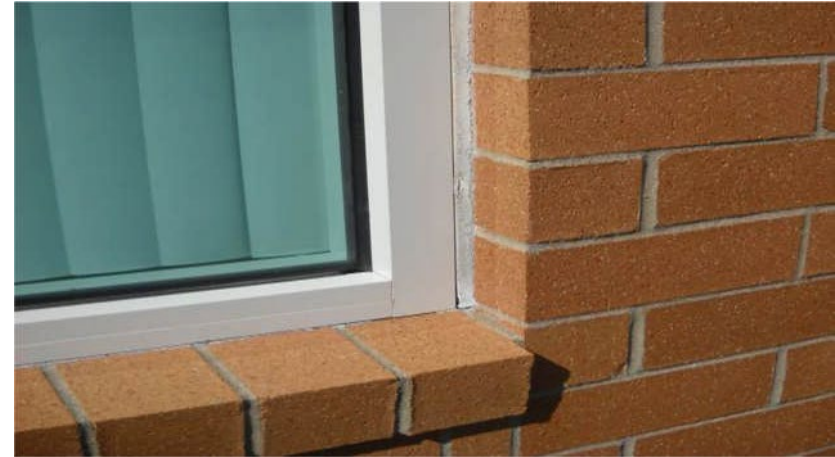
Health Education Building – Typical sealant joint is at end of life.
