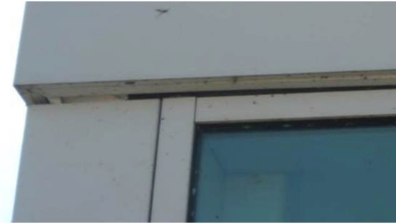
La-Z-Boy Center – It appears there is a void within the exterior aluminum, curtain wall assembly allowing the environment to enter the interior.
