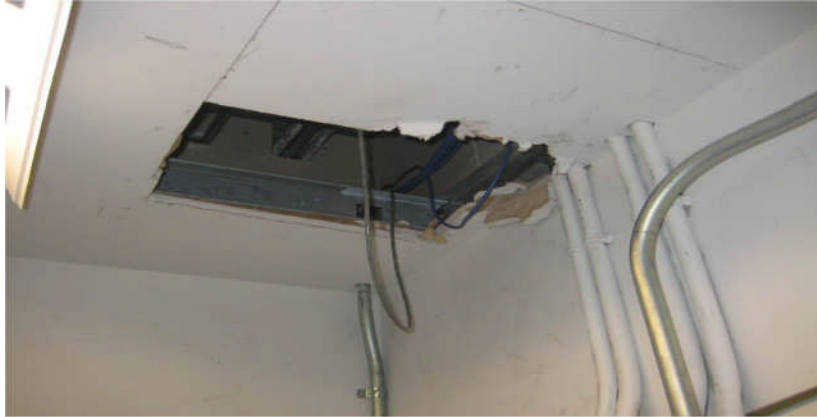
Whitman Center – breach in fire-rated ceiling assembly.
