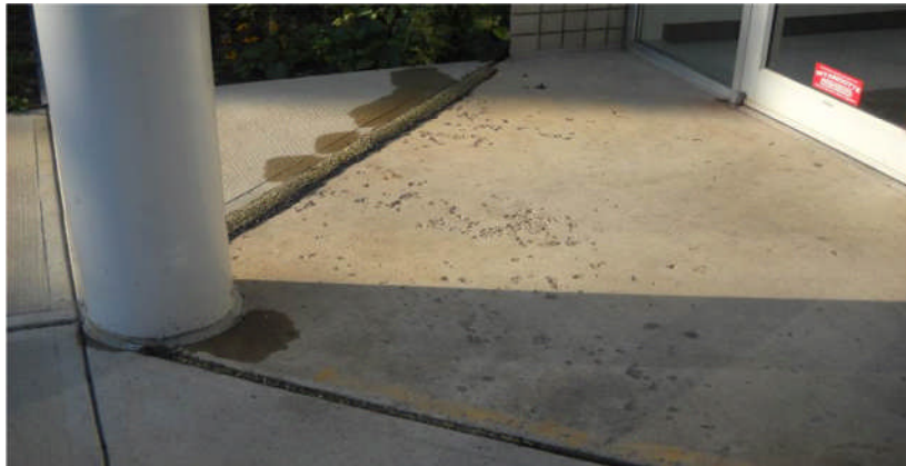
Whitman Center – settlement/heaving of exterior concrete slab (at main entrance) presents a tripping hazard.
