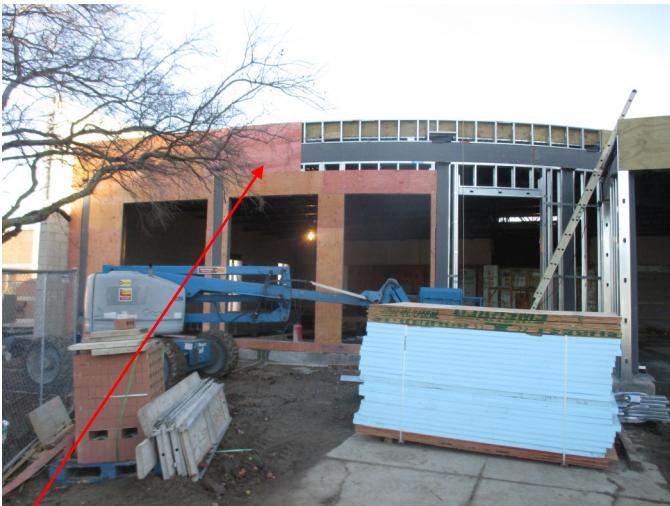
The top-left photo shows the progress of the installation of the plywood sheathing on the exterior side of the curved west wall of the addition. Once the sheathing is finished and covered with a vapor barrier the brick veneer can be installed.
