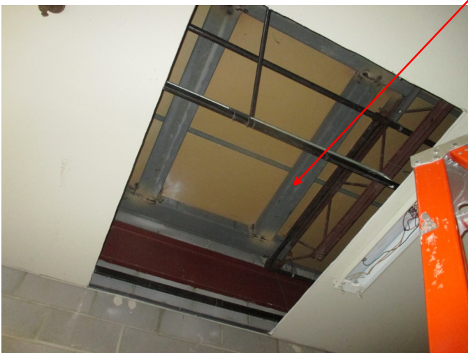
The bottom-left photo shows the installation of the support steel for the new roof access hatch for the roof over the north wing of the existing building. Previously this roof was only accessible by ladder, however when the access hatch is finished the maintenance staff will be able to gain access to the roof without the need for a ladder.
