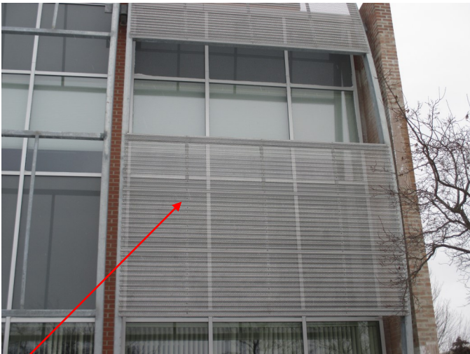
The top-left photo shows the first of the corrugated mesh panels installed that will help serve as shades on the northwest face of the building.
