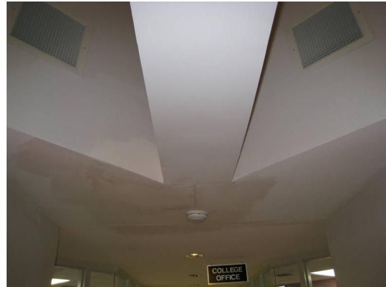
Whitman Center – College is completing repairs to ceiling damage and has installed movement joints in an effort to limit future cracking. The lack of movement joints is causing cracking elsewhere in the facility.
