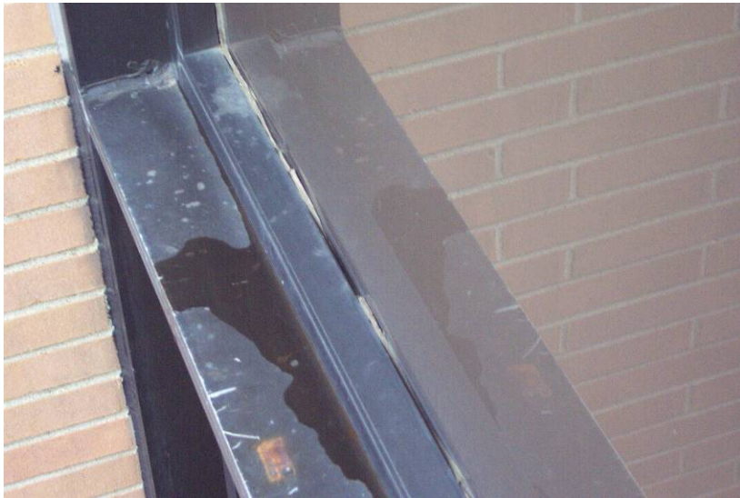
Life Sciences Building – failing original sealant allowing water infiltration, causing damage to interior finishes.
