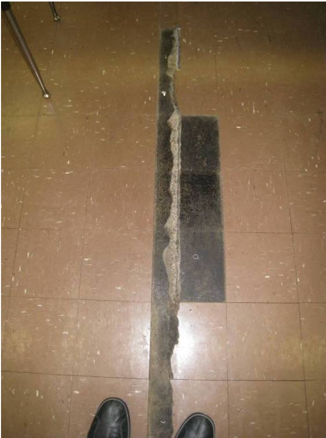
West Technology – concrete slab movement has telegraphed through the floor tile resulting in a failed section of flooring.
