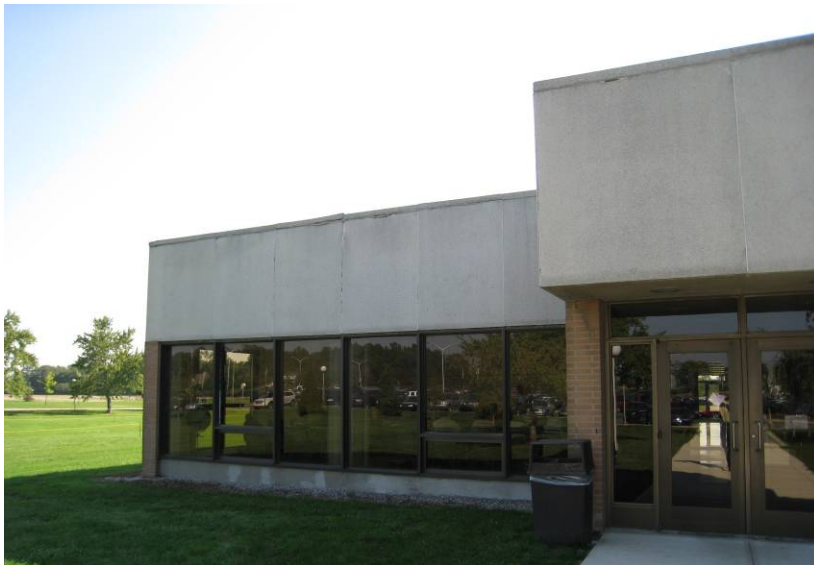
Life Sciences Building – concrete composite parapet caps loose, cupping and deteriorating.
