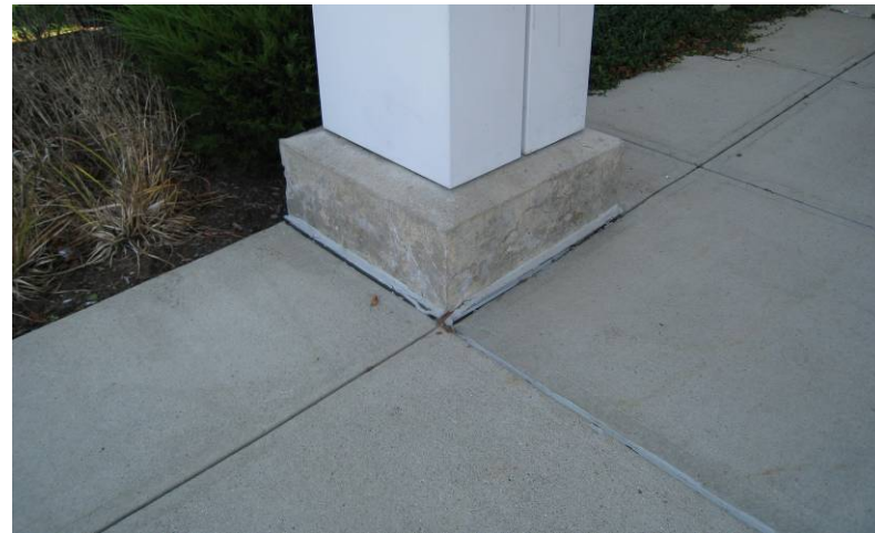
Health Education Building – settlement in exterior slabs may result in a tripping hazard and should be monitored.
