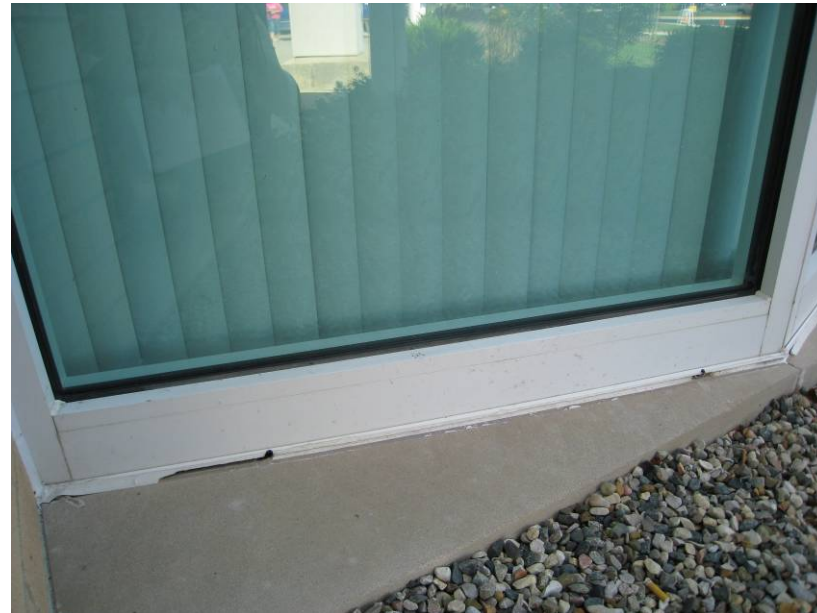
Health Education Building – Ongoing water infiltration problems with the aluminum window framing should be monitored.
