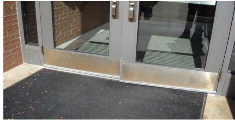
Student Services/Administration - Aluminum entrance doors and hardware at end of life.
