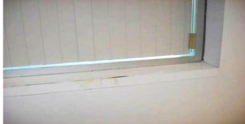
Whitman Center – water infiltration along exterior wall has caused deterioration of the plastic-laminated windowsills.
