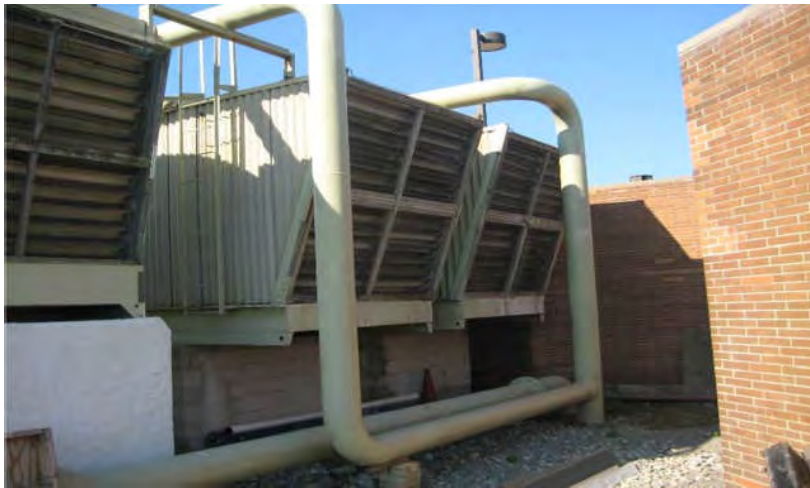
Physical Plant – Cooling tower and basins are near end of life.
