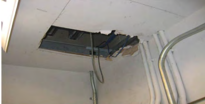
Whitman Center – breach in fire-rated ceiling assembly.
