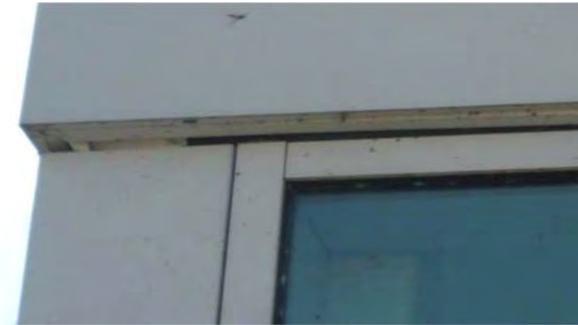
La-Z-Boy Center – It appears there is a void within the exterior aluminum, curtain wall assembly allowing the environment to enter the interior.
