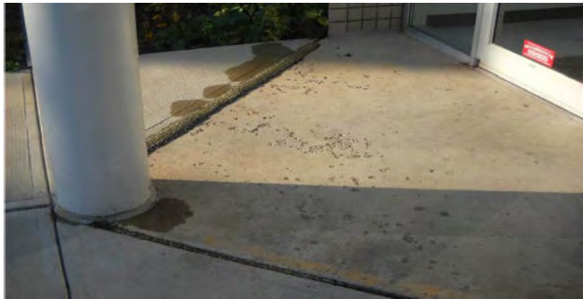
Whitman Center – settlement/heaving of exterior concrete slab (at main entrance) presents a tripping hazard.
