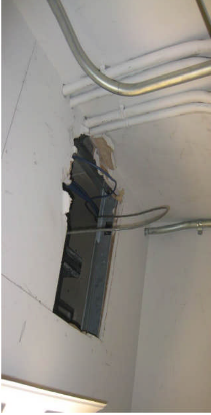
Whitman Center – breach in fire-rated ceiling assembly.
