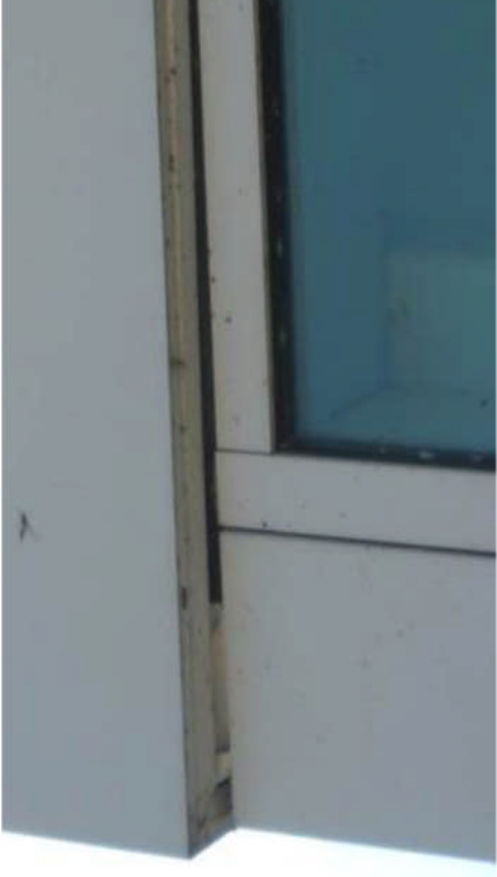
La-Z-Boy Center – It appears there is a void within the exterior aluminum, curtain wall assembly allowing the environment to enter the interior.
