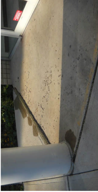
Whitman Center – settlement/heaving of exterior concrete slab (at main entrance) presents a tripping hazard.
