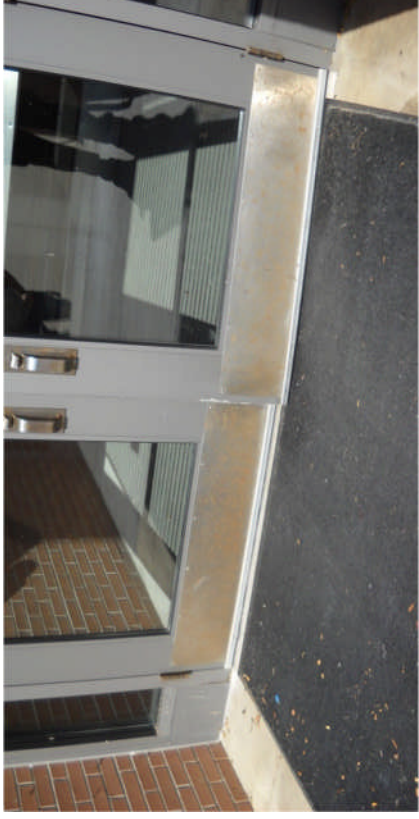
Student Services/Administration - Aluminum entrance doors and hardware at end of life.
