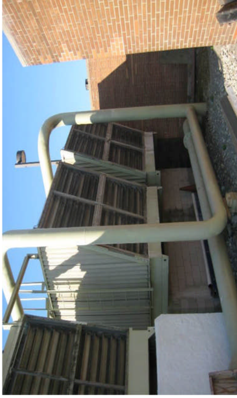
Physical Plant – Cooling tower and basins are near end of life.
