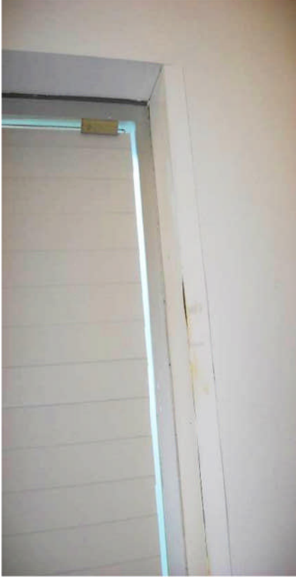
Whitman Center – water infiltration along exterior wall has caused deterioration of the plastic-laminated windowsills.
